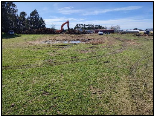
Photo 3: Standing water in centre of site.
